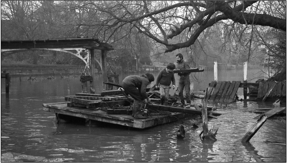
Volunteers clear away rotten timbers from the bridge deck near the island
