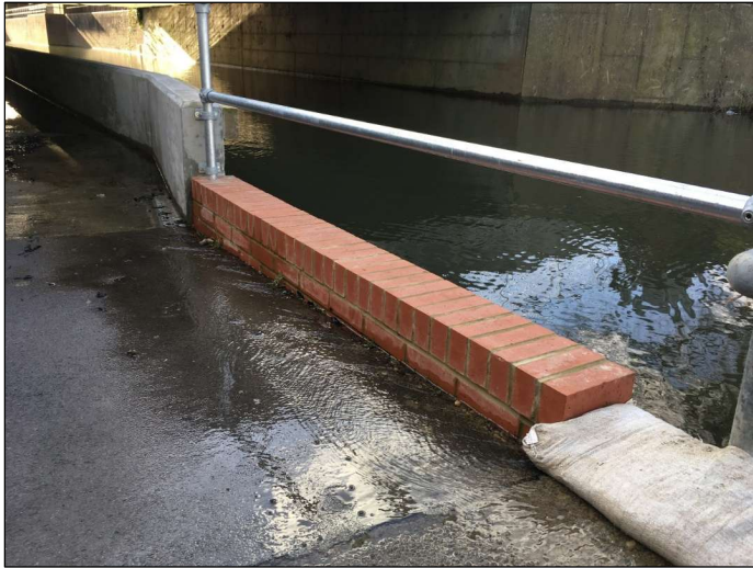
The new brick wall, as at 18 th January 2018 - already watery!
